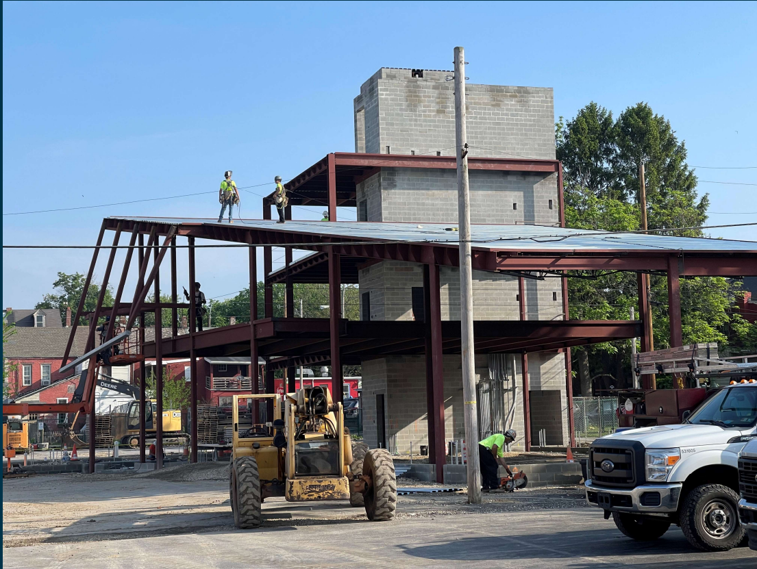
Stewart and Tate Construction personnel can be seen working on the under-decking for the roof of the CAY HCC Orr Event Hall.
